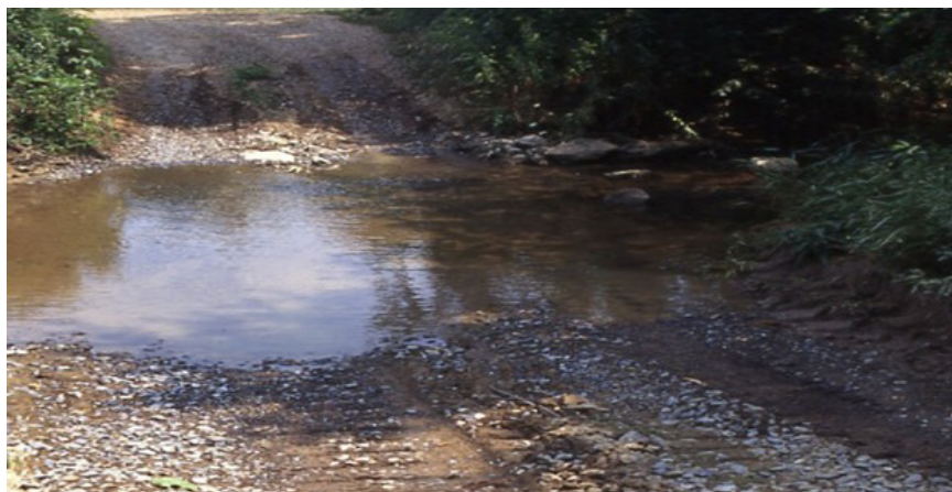
Figure 8b. Correctly Constructed Ford
