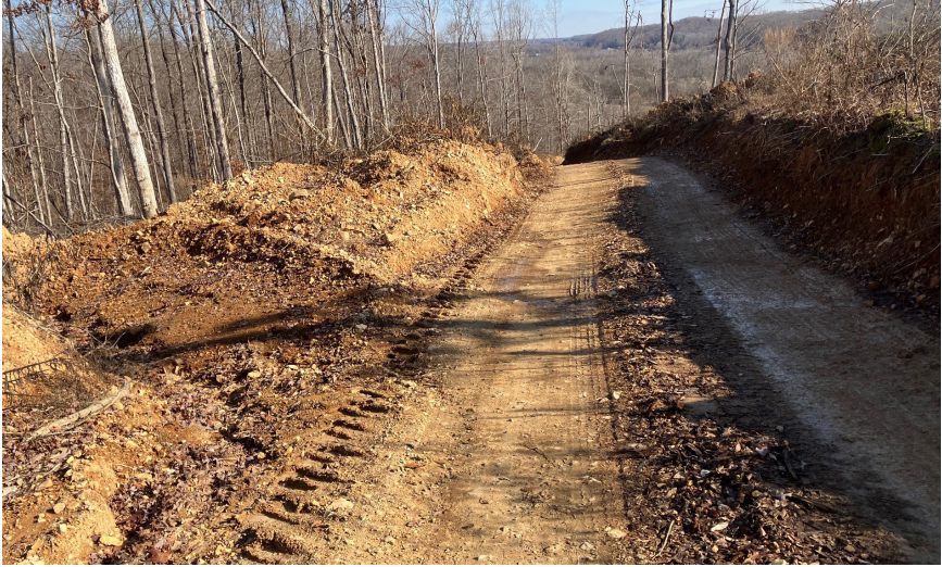
Figure 3. Main log road with turn out.
