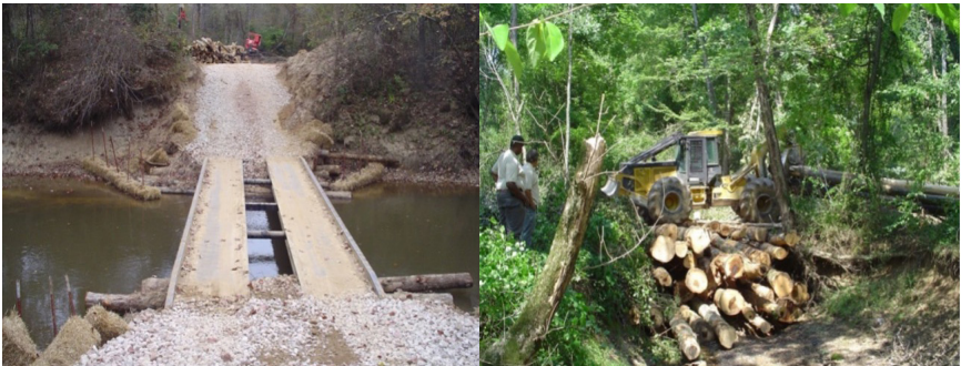
Figure 10. (left) Portable steel bridge suitable for hauling. (right) Temporary pole bridge suitable for skidding and hauling. Temporary bridge structures should be removed after use.
